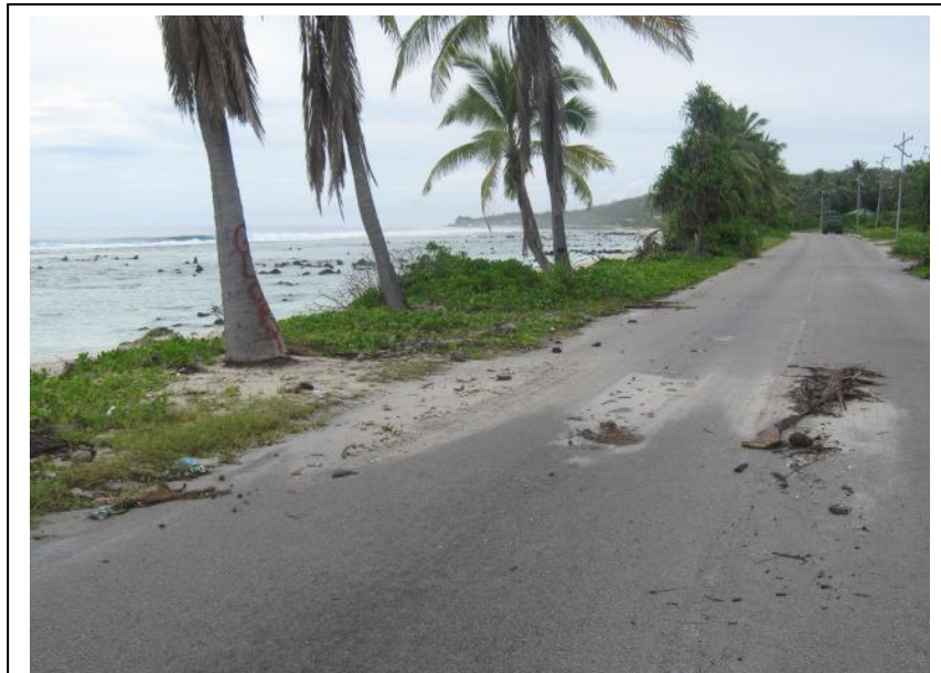
ANIBARE BEACH COASTLINE BEARING SIGNS OF DEBRIS FROM OVERTOPPING KINGTIDES
